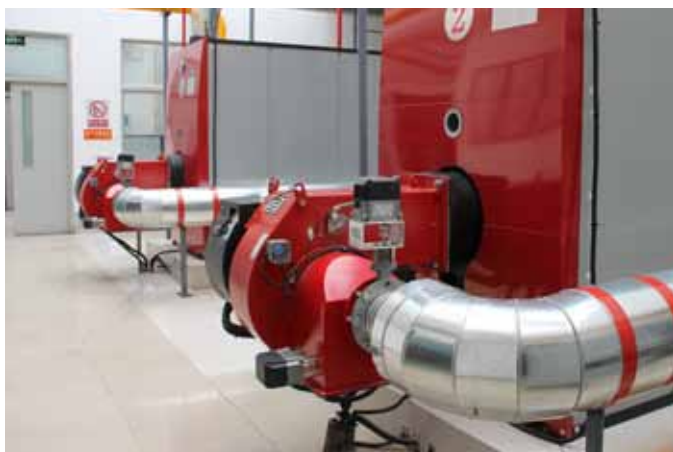
2x BLU 4000 FGR mounted on 2x 2,8 MW hot water boiler units
