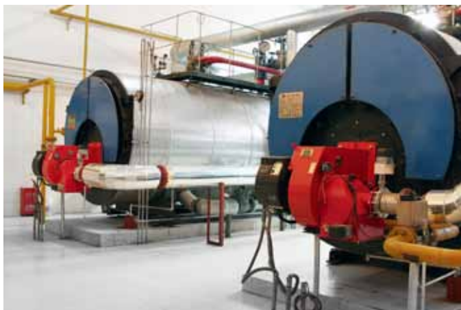
2x BLU 6000 FGR mounted on 2x 4,2 MW hot water boiler units
