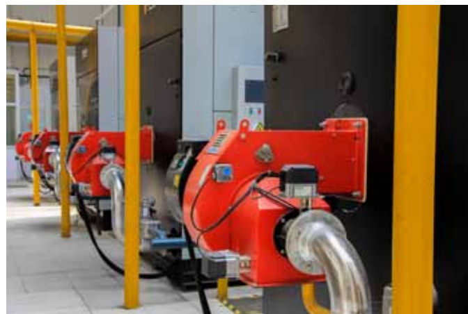
4x BLU 4000 FGR mounted on 4x 2,8 MW hot water boiler units
