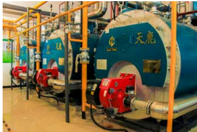
3x BLU 3000 FGR mounted on 3x 1,4 MW hot water boiler units
