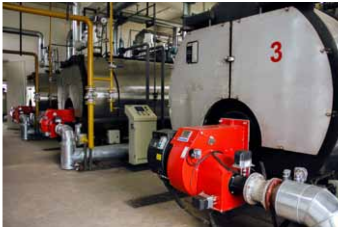
3x BLU 4000 FGR mounted on 3x 4 TPH steam boiler units
