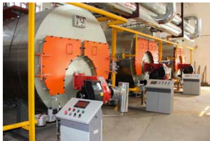
2x BLU 4000 FGR on 2x 2,8 MW hot water boilers 1x BLU 2000 FGR on a 1,4 MW hot water boiler
